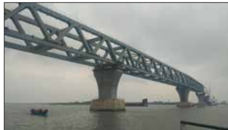
Full length of Padma bridge is now visible with the installation of 41th span
